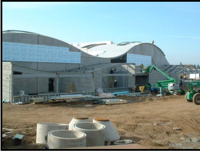
Workers placing steel roof supports over the main entry way and applying roof coving over the gymnasium.
